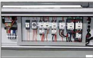
Electrical Control Box
